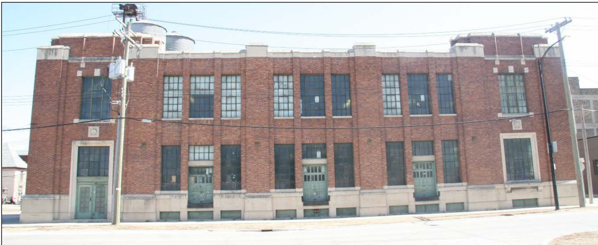
Plate 14 – T. Eaton’s Company Printing Plant & Track Warehouse, 130 Galt Avenue, west façade, 2015. ( M. Peterson, 2015. )
