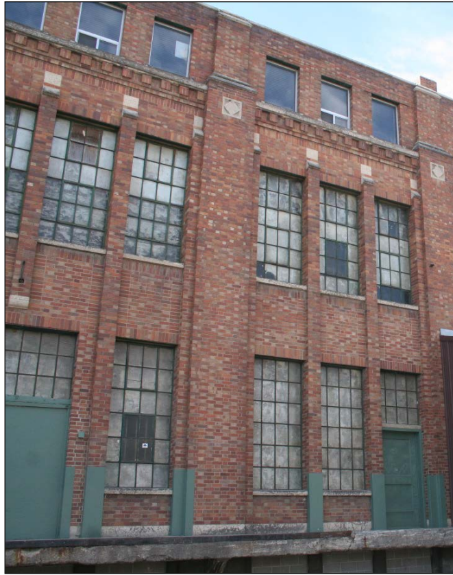
Plate 11 – T. Eaton’s Company Printing Plant & Track Warehouse, 130 Galt Avenue, window details, north side (east end), 2015. ( M. Peterson, 2015. )
