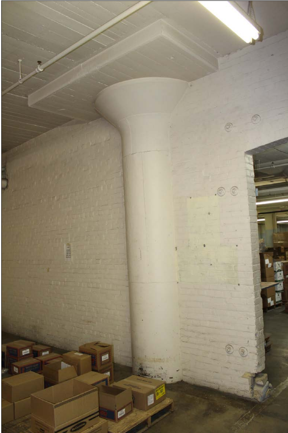
Plate 22 – T. Eaton’s Company Printing Plant & Track Warehouse, 130 Galt Avenue, 1927 building, basement concrete beams and brick interior dividing wall, 2017. ( M. Peterson, 2017. )
