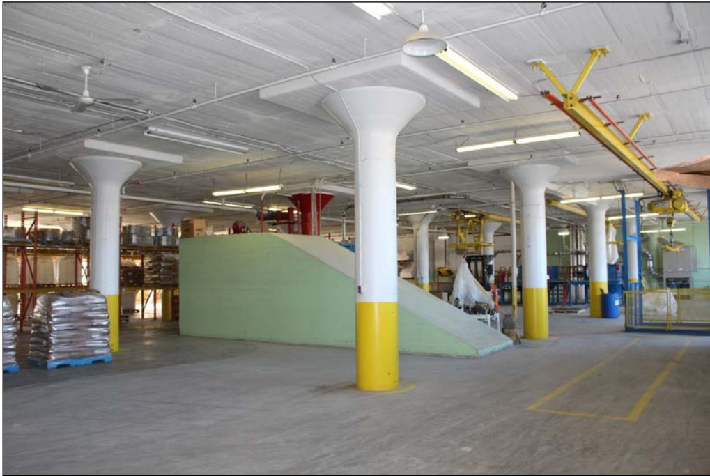
Plate 20 – T. Eaton’s Company Printing Plant & Track Warehouse, 130 Galt Avenue, 1926 building, second floor, 2017. ( M. Peterson, 2017. )
