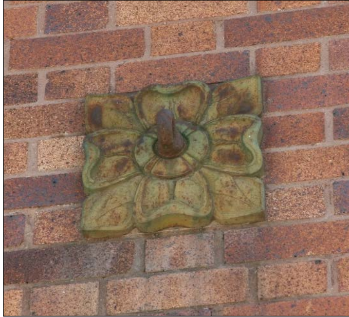
Plate 18 – T. Eaton’s Company Printing Plant & Track Warehouse, 130 Galt Avenue, floral detail on west façade, 2015. ( M. Peterson, 2015. )
