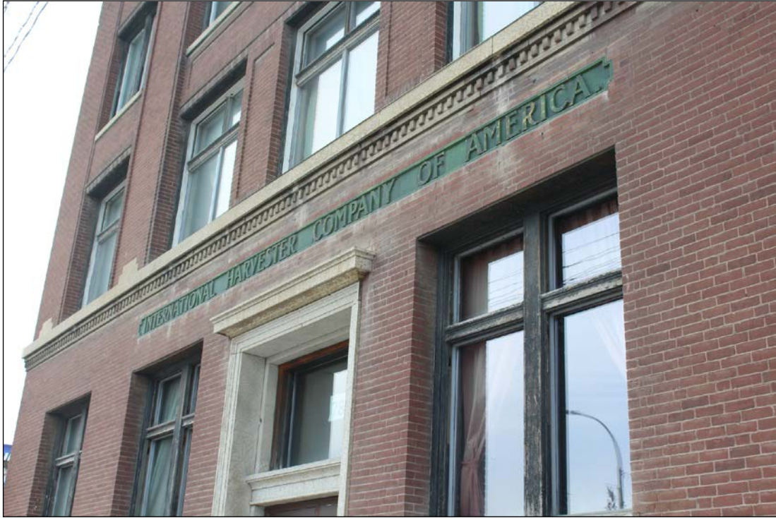
Plate 10 – International Harvester Building, 782 Main Street, detail of front (east) façade, 2017. ( M. Peterson, 2017. )
