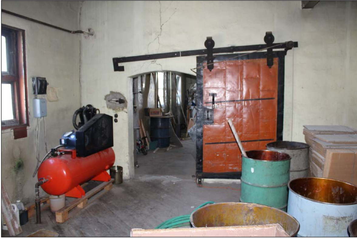
Plate 14 – Scott-Bathgate Building, 149 Pioneer Avenue, 5 th floor connecting doorway with metal-clad fire door, 2017. ( M. Peterson, 2017. )
