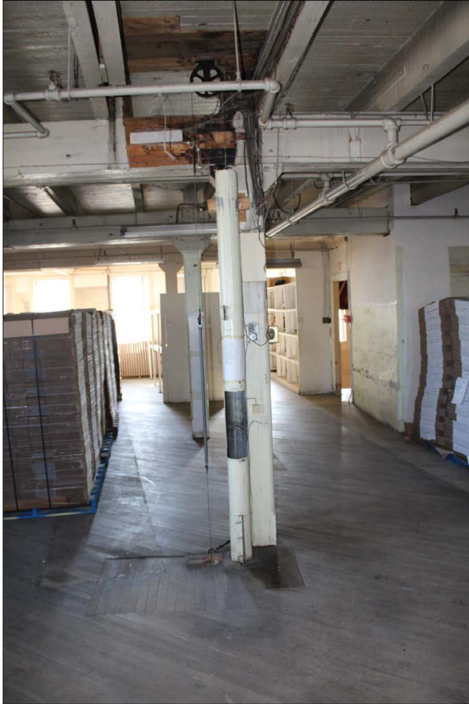
Plate 16 – Scott-Bathgate Building, 149 Pioneer Avenue, top of the tube messaging system, 3 rd floor, 2017. (M. Peterson, 2017.)
