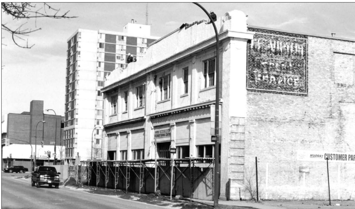
Plate 23 – McLaughlin-Buick Garage, 275 Maryland Street during 1999 demolition; built 1909, architect J.D. Atchison, front (west) façade. (D.M. Lyon, 1999.)
