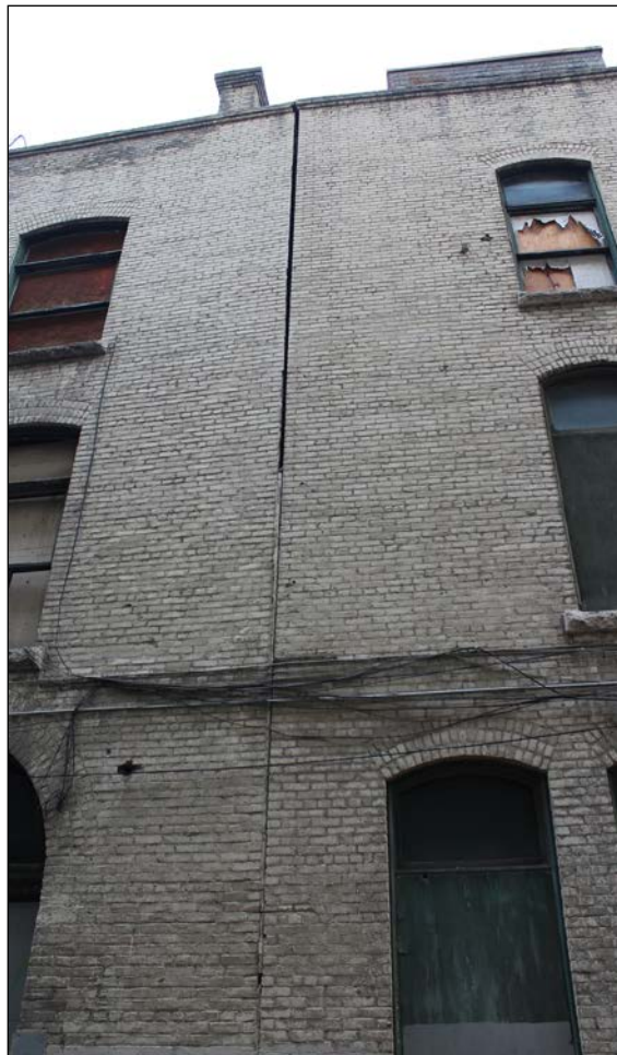
Plate 8 – McLaughlin Carriage Company Building, 208 Princess Street, cracks in the front (east) and rear (west) façades, 2015. (M. Peterson, 2015.)
