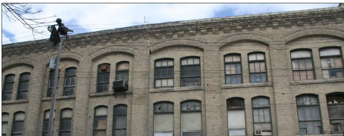
Plate 10 – McLaughlin Carriage Company Building, 208 Princess Street, detail of front (east) façade, 2015. (M. Peterson, 2015.)
